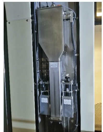
Tank and pumps
